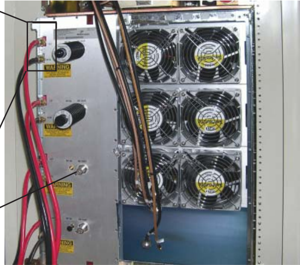
Fig. 3-13, DC Integration Cable
