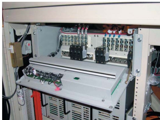
Fig. 3-12, DC Breaker Panel
