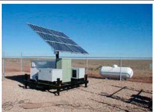
Alpha Energy HPS24-1050/1500-2GEN in Amarillo, Texas.
