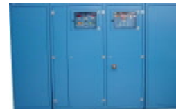
3500A Rectifiers "PIRELLI" Steel Chord Plants
