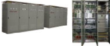
110VDC Rectifiers 30kVA 1Ph. Inverters "IRASCO" Refineries—Iran
