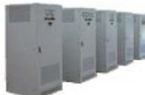
110/220VDC Rectifiers 30kVA 1Ph. Inverter "GENERAL ELECTRIC" Port Talbot—UK
