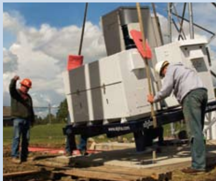
Hybrid Power System (HPS) with solar, generator and battery power
