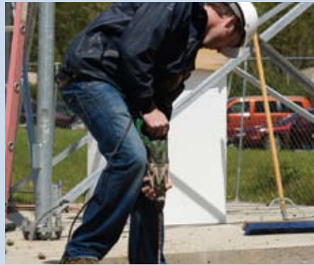
Comprehensive design, engineering and installation capabilities
