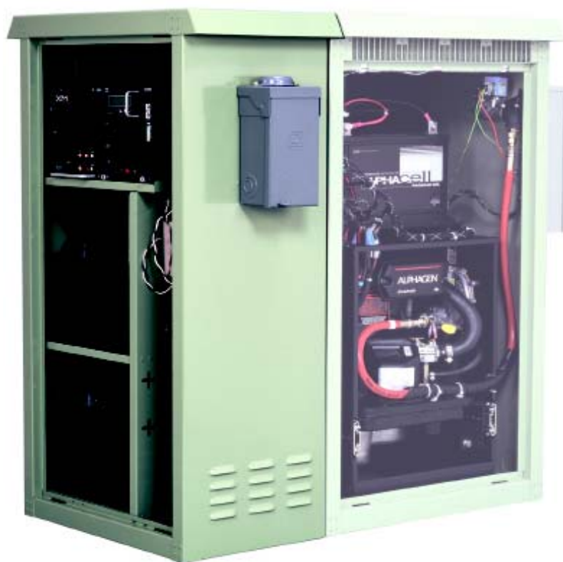
Fig. 1 Sidecar and Generator Enclosure
