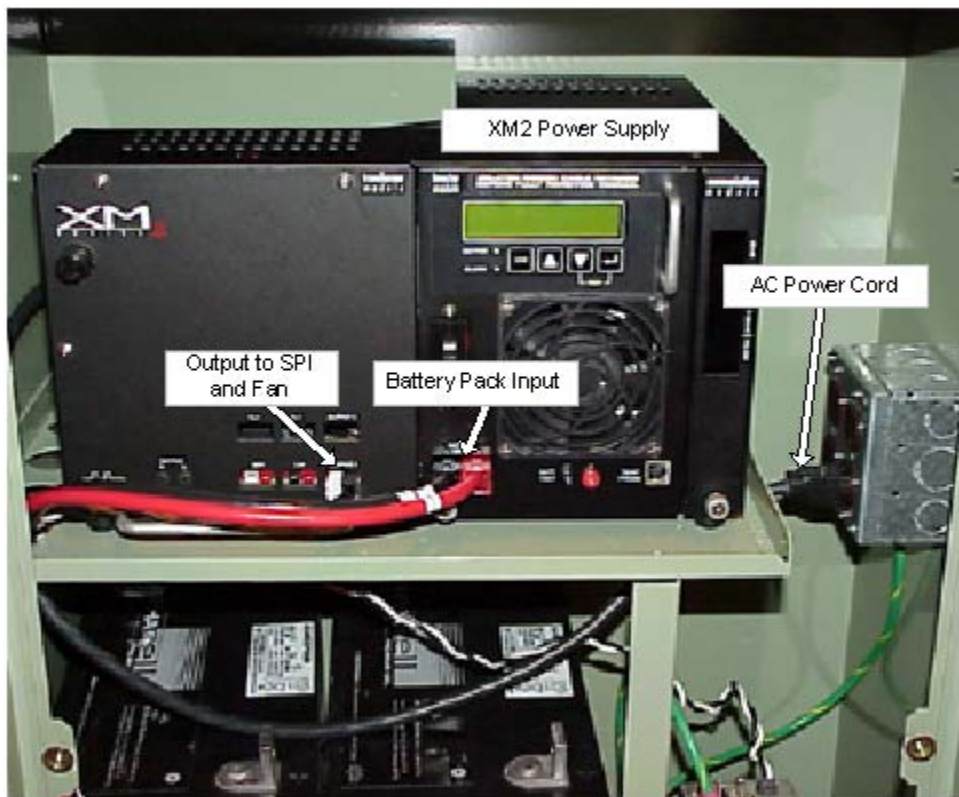
Fig. 9 Power supply on Shelf
