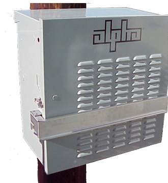
Fig. 10, Security Device Installed
