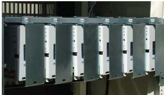
Figure 18–Six rack mounted FMPS power modules
