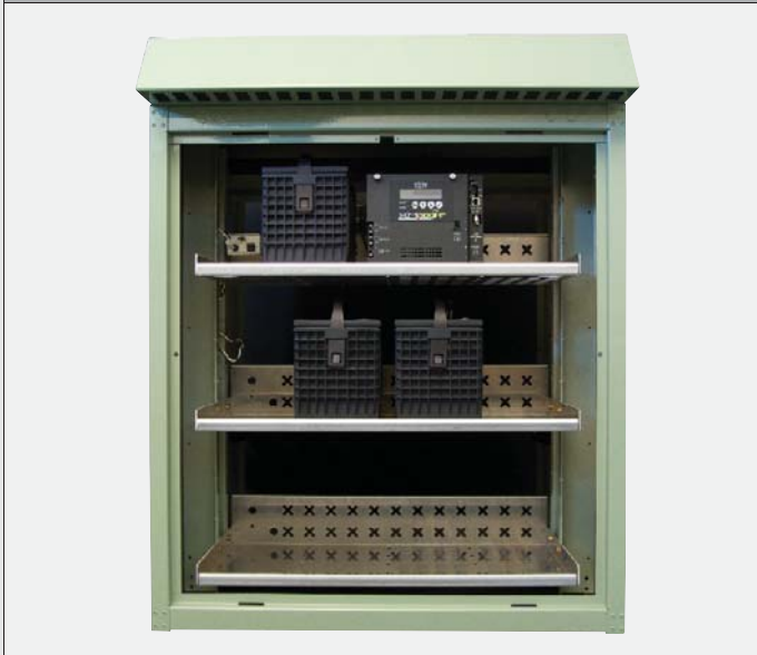
XM2-300HP, 1 AlphaCell Battery and 2-Battery Back-up Pack
