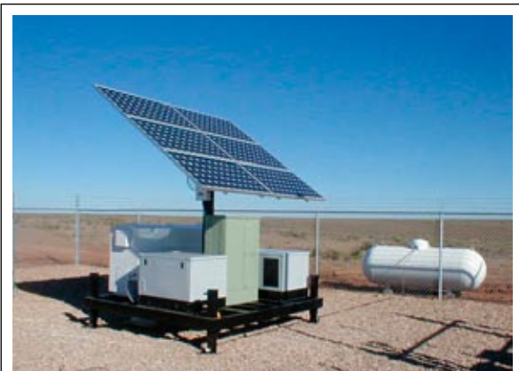
Alpha Energy HPS24-1050/1500-2GEN in Amarillo, Texas.
