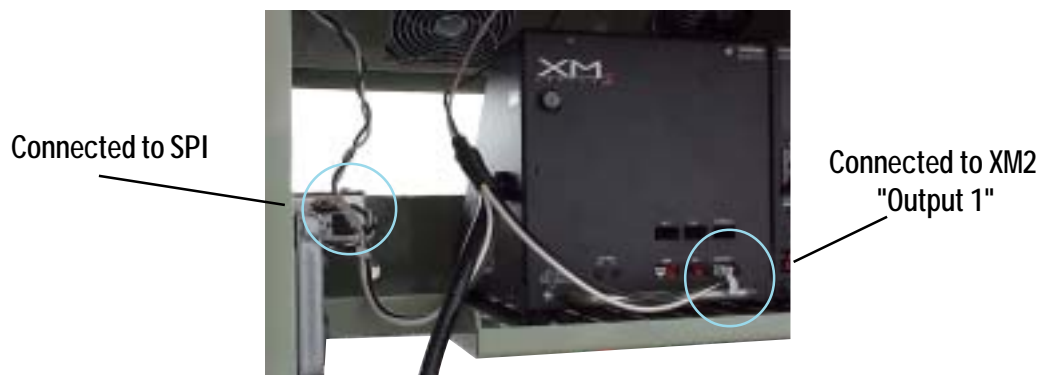
Figure 4-16; Cooling Fan Plugged into Power Supply and SPI
