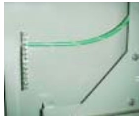
Figure 3-12; SPI Ground Wire Connected to Enclosure Ground Bar
