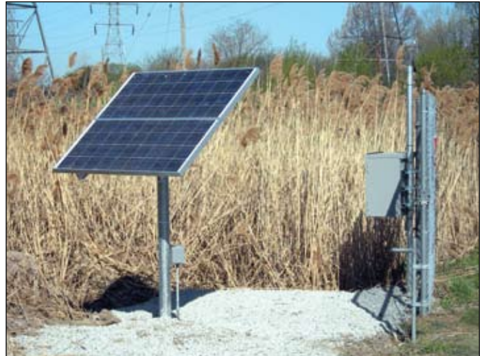
Alpha Energy New York SPS Installation.
