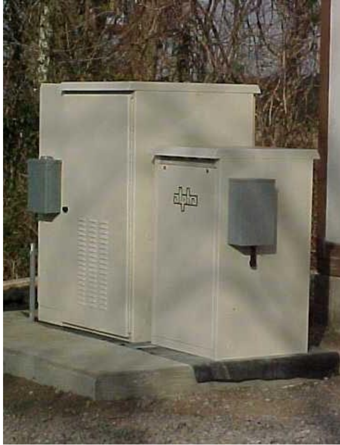
Figure. 4. Installed telecom genset collocated with RT. Genset is the smaller enclosure on the right of the figure.
