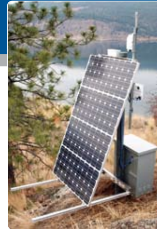
Wi-Fi Solar Power System
