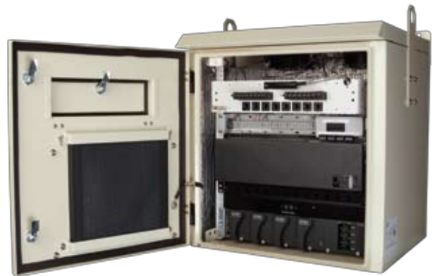
Fiber Backhaul Enclosure
