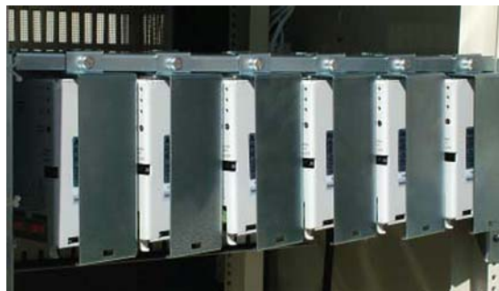
Figure 18–Six rack mounted FMPS power modules
