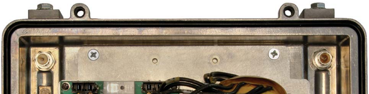
Fig. 2-5, RF Module Removed
