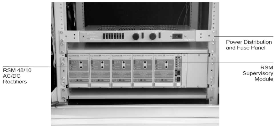
Rectifier kit with stand-alone fuse panel in a controlled environment Remote Terminal
