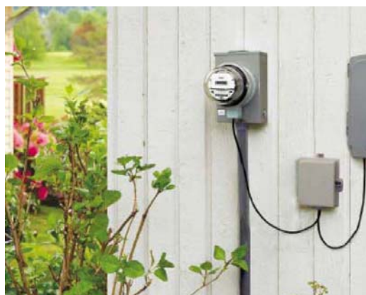
AC to DC power converter installed in a socketed meter collar and an 18 Watt battery module supporting the ONT at the home
